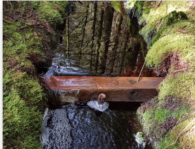
Timber dam in a small drain, draining a Forest Service NI compartment.
